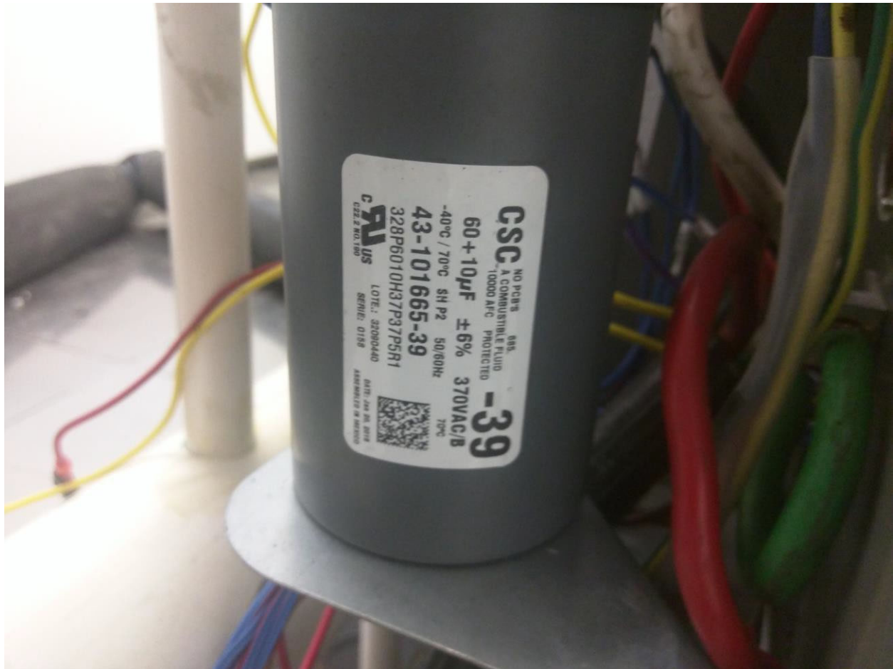
Outdoor unit - capacitor
