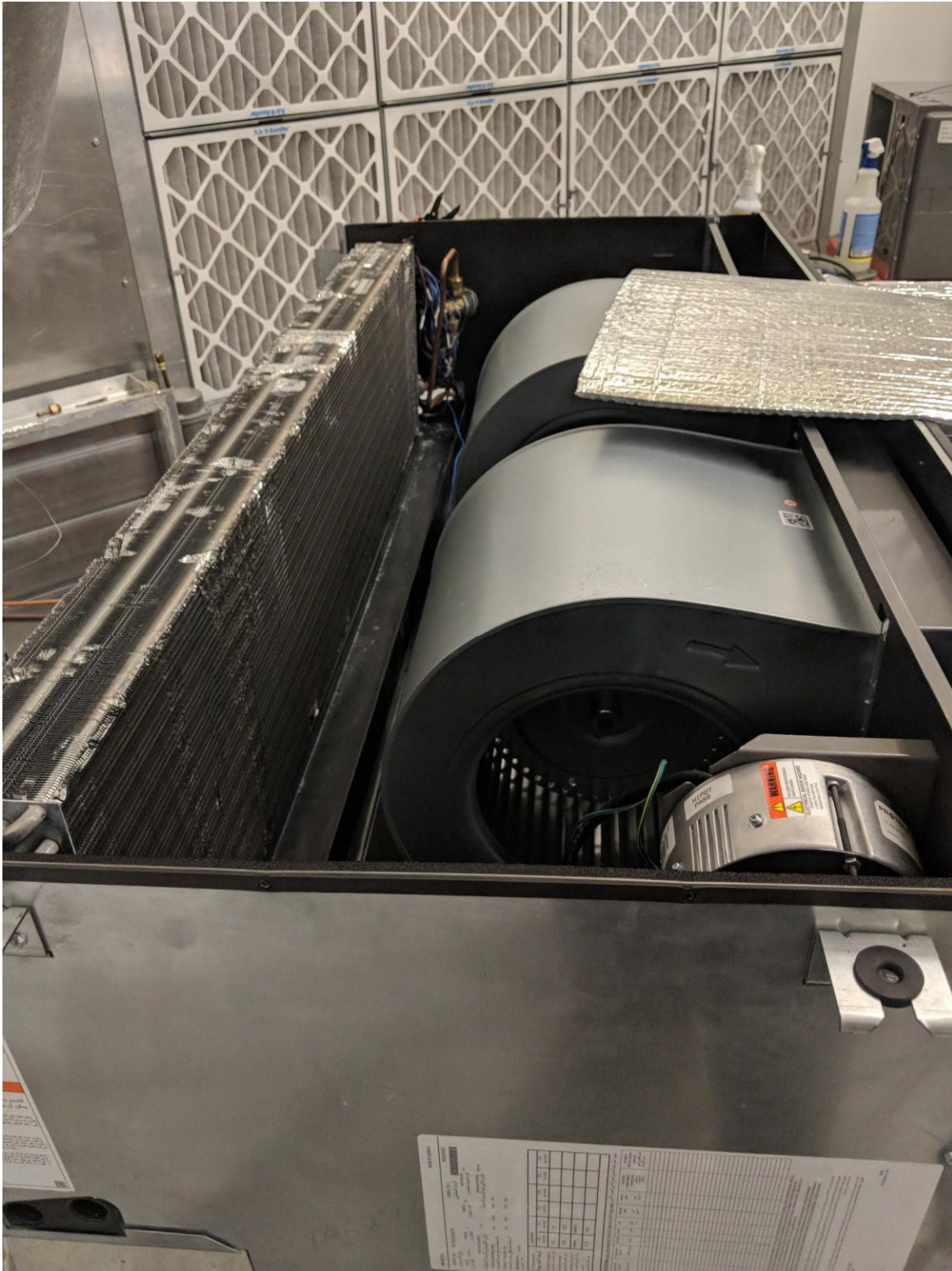
Indoor unit - motor compartment
